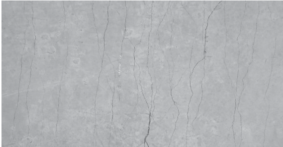
FIG. 3. Multiple cracking along the length of the specimen.
