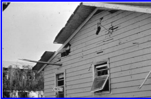
Fig. 3.6: Windborne debris can often generate dangerous missiles.
