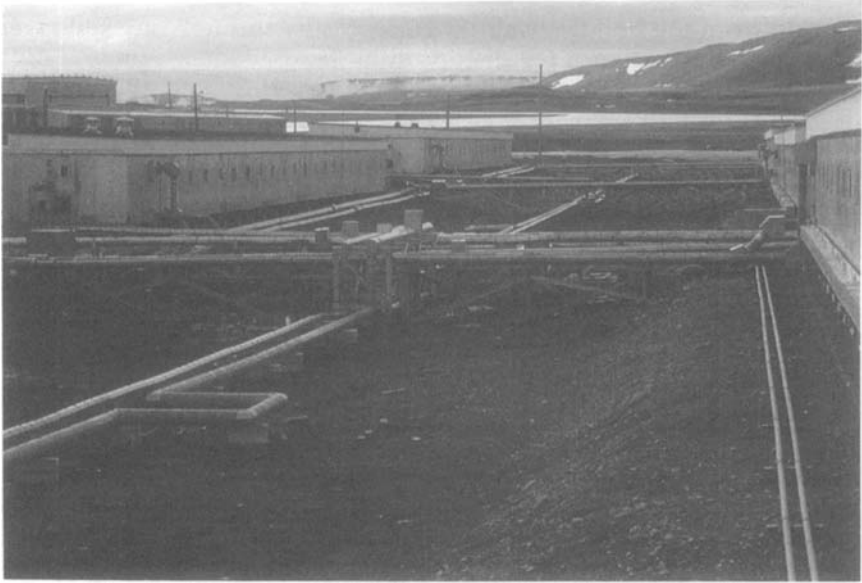
FIG. 10.9 Utilidor System Can Create an Unappealing Complex of Pipes (CRREL photo, D. R. Freitag)
