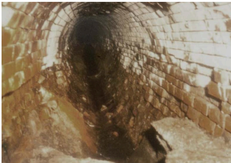
Figure F.16 — Example of missing mortar
