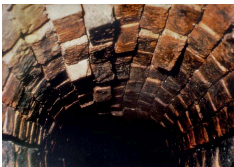
Figure F.12 — Example of collapse
