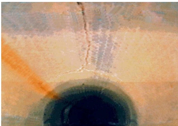
Figure F.30 — Example of lining defect (longitudinally wrinkled lining)
