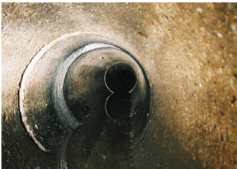
Figure F.26 — Example of displaced joint (radial)
